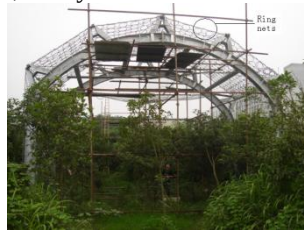
Fig.2 Flexible rock-shed including ring nets and steel vaulted structure
