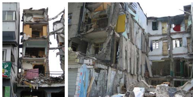
Fig. 5 Failure due to horizontal dynamic loading
