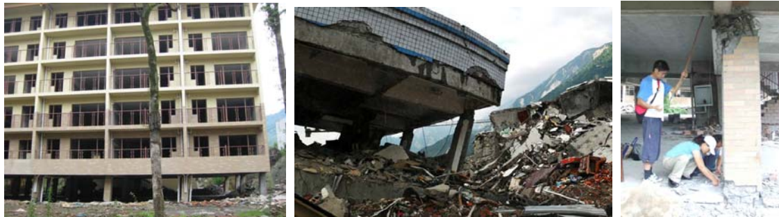
Fig. 4 Soft storey failure
